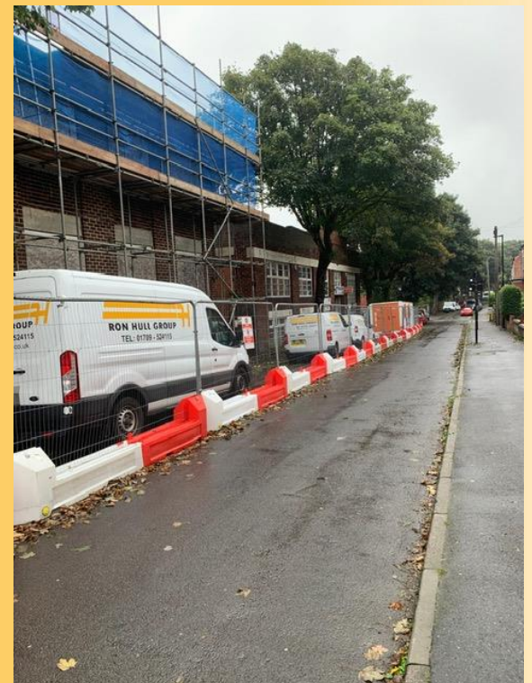
Footpath and half road closure in effect along Cliffe Road for full demolition duration
